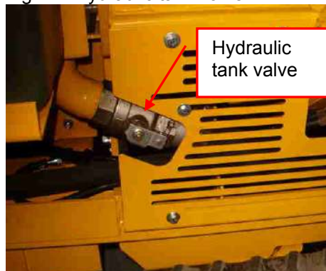
Fig 4.1 Hydraulic tank valve
